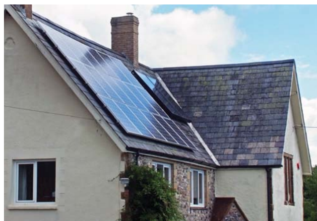
PV and solar panels installed on an older property
