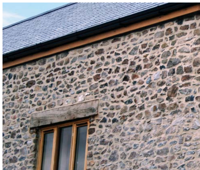
The most characteristic construction material in the Blackdown Hills is chert
